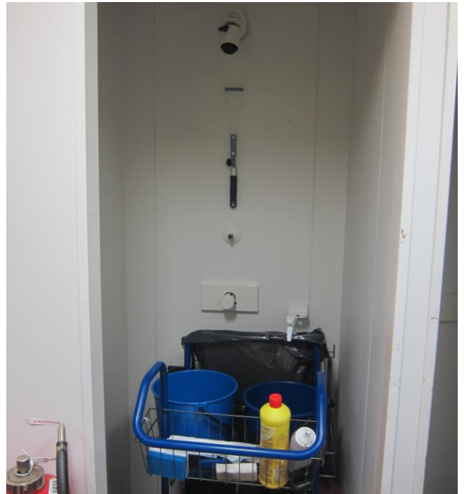
Figure 9.11: This shower is not in use, and is used for storage. Water in such pipes will be at room temperature, and there is a growth potential for Legionella and other microbes. This water may then contaminate the rest of the piping. Piping that is not in use should be eliminated, alternatively flushed weekly (Photo: Eyvind Andersen)
