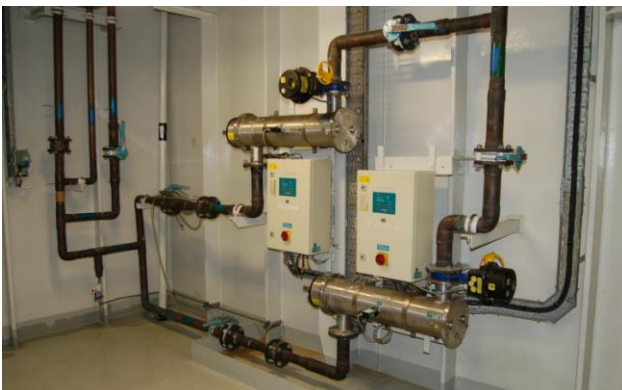
Figure 8.5: This UV-unit has two radiation chambers, each chamber has a control panel (white) and an UV-sensor (on the front). The black valve closes if the radiation falls below the alarm level. (Photo: Eyvind Andersen)
