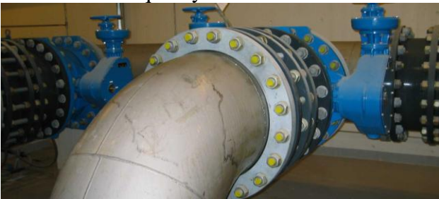
Figure 9.16: Pipes and valves in potable water systems vary in size and material. It is important that corrosion resistant materials and materials that do not encourage bacterial growth are chosen (Photo: Eyvind Andersen)
