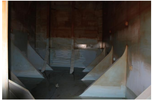
Figure 5.3: This potable water tank is high and lacks internal platforms for easy cleaning. This has resulted in insufficient cleaning. The walls are pretty clean up to 2 meters height and very dirty above 4 meters height (Photo: Eyvind Andersen)
