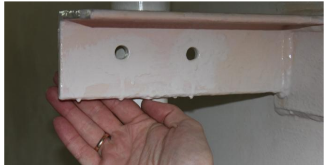
Figure 9.9: Picture from a tank where wrongful coating application has resulted in corrosion and need for touch ups. Coating applied to thickly on cold steel and by wrong application methods, increase the risk for growth of micro-organisms, as well as problems with unpleasant smell and taste from tank coating (Photo: Eyvind Andersen)
