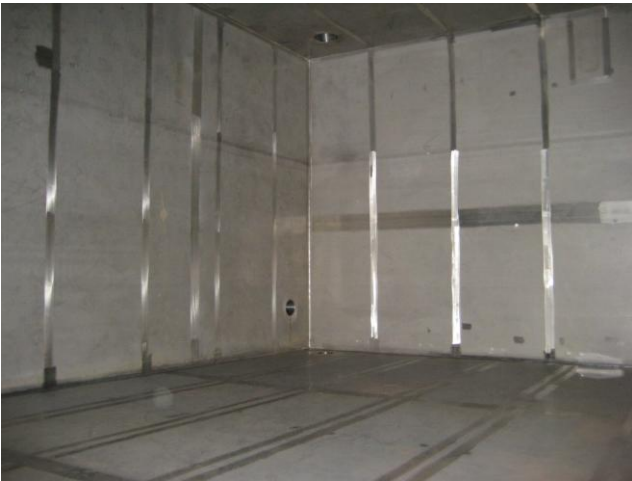
Figure 9.1: Approximately 4 meters high potable water tank in stainless steel with no obstructing internal structures. Such tanks are easy to clean, and problems with applying and maintenance of coating is avoided (Photo: Bjørn Løfsgaard)
