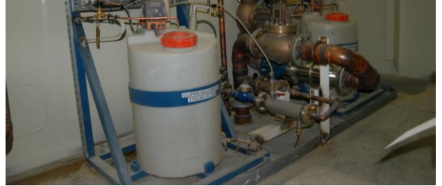
Figure 5.7: A marked and protected chlorine tank with easy access (Photo: Eyvind Andersen)
