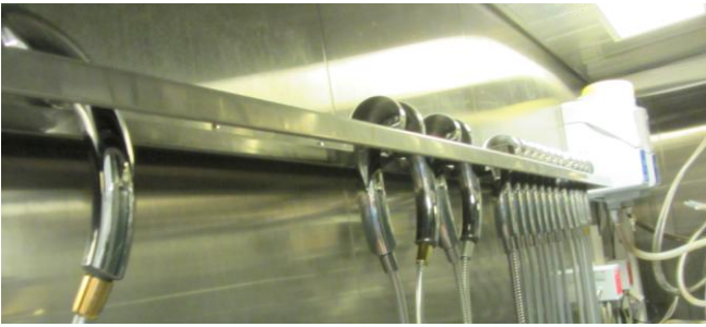
Figure 9.18: Shower hoses and heads are problem spots for Legionella growth due to low temperatures after mixers combined with stagnant water when not in use. Here growth is prevented through drying of the equipment (Photo: Arild Tolo)
