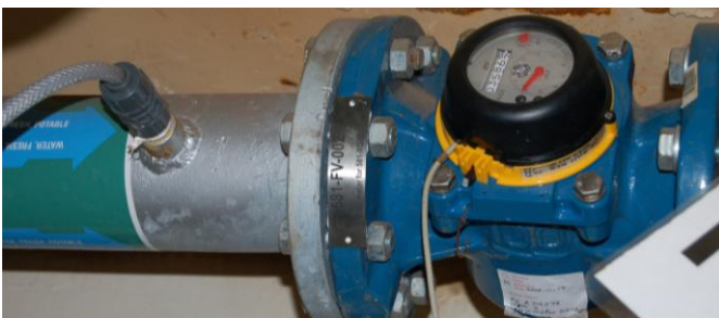
Figure 7.6: The flow meter display is visible to the right, and the chlorine hose and dosing point to the left (Photo: Eyvind Andersen)
