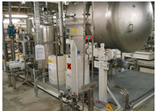
Figure 1.1: Potable water system with evaporator, scale inhibitor tank, chlorine tank, alkalizing filter and UV-units (Photo: Eyvind Andersen)
