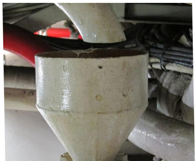
Figure 9.12: Full air gap of type «AA» is the best way of eliminating contamination from other systems supplied with potable water (Photo: Eyvind Andersen)
