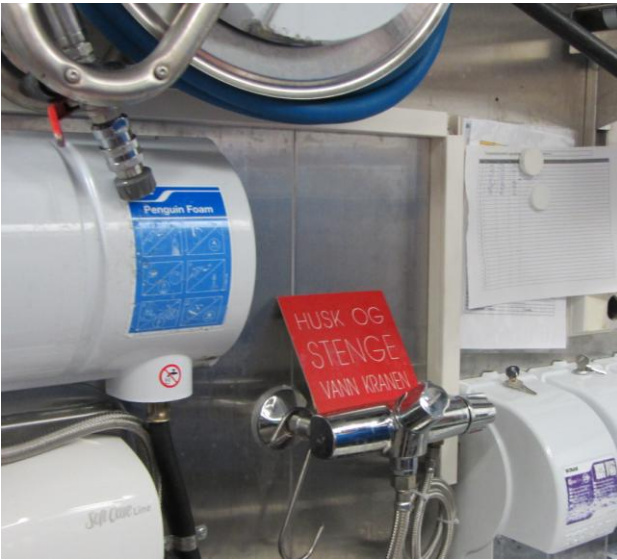
Figure 9.15: A hose station where water is leaking between the hot and the cold water when the mixer is left in open position and the hose is not in use. A sign to close the mixer is not a barrier against such leaks (Photo: Eyvind Andersen)
