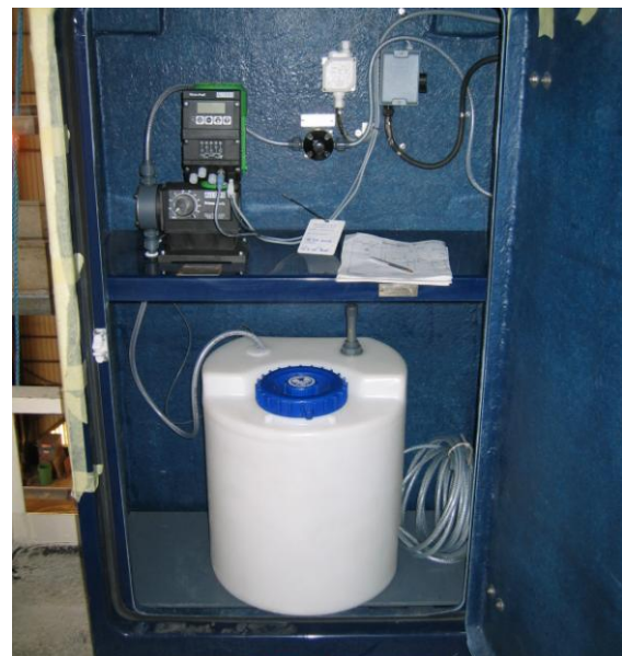
Figure 8.3: Flow meter controlled chlorination unit, safely placed in a cabinet (Photo: Bjørn Løfsgaard)
