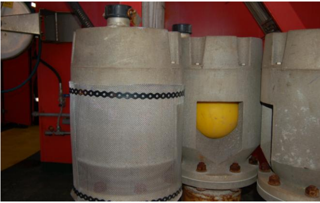
Figure 9.3: Air vents for potable water tanks must be sufficiently protected. The picture shows vent safeguarded with floating ball and fine mesh corrosion material. The picture is taken on a newbuild prior to marking (Photo: Eyvind Andersen)
