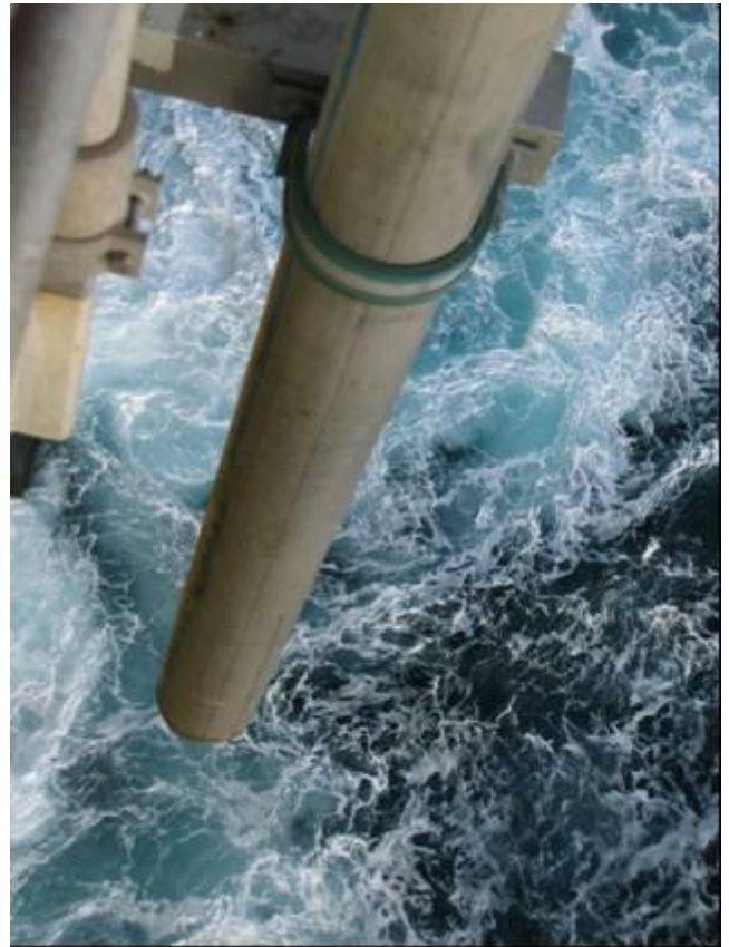
Figure 7.8: When flush valve and the bunkering hose have corresponding diameters the system can be flushed with maximum pressure. (Photo: Eyvind Andersen)
