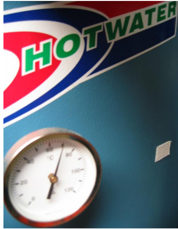
Figure 9.17: Legionella can be prevented by keeping the cold water cold and the warm water warm (Photo: Eyvind Andersen)
