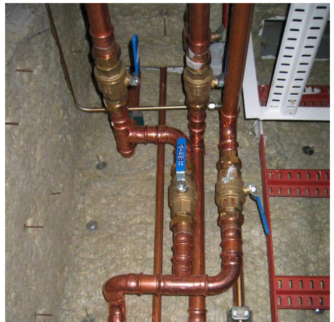
Figure 4.7: Corrosive water in copper pipes can result in too high copper content in the potable water (Photo: Bjørn Løfsgaard)
