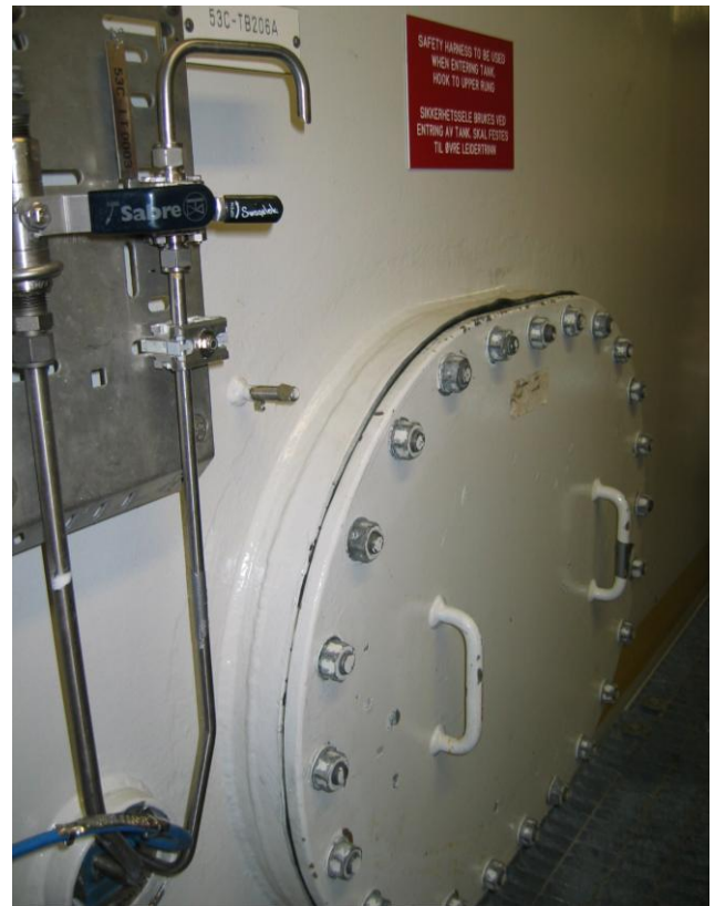
Figure 9.4: The picture shows a storage tank with easily reached test tap and an accessible manhole (Photo: Eyvind Andersen)
