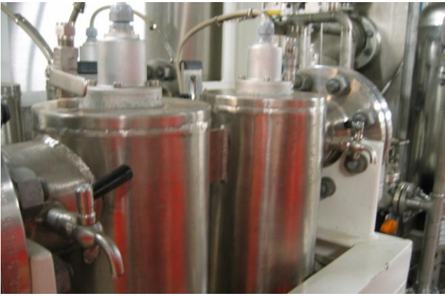
Figure 8.7: UV-unit with test taps before and after disinfection (Photo: Eyvind Andersen)
