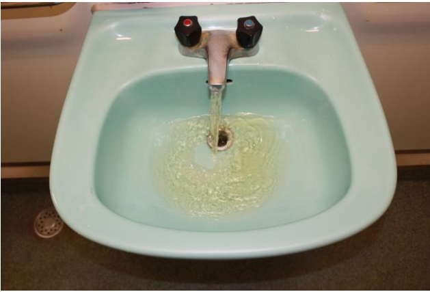
Figure 4.3: Discoloured water due to corrosion (Photo: Eyvind Andersen)
