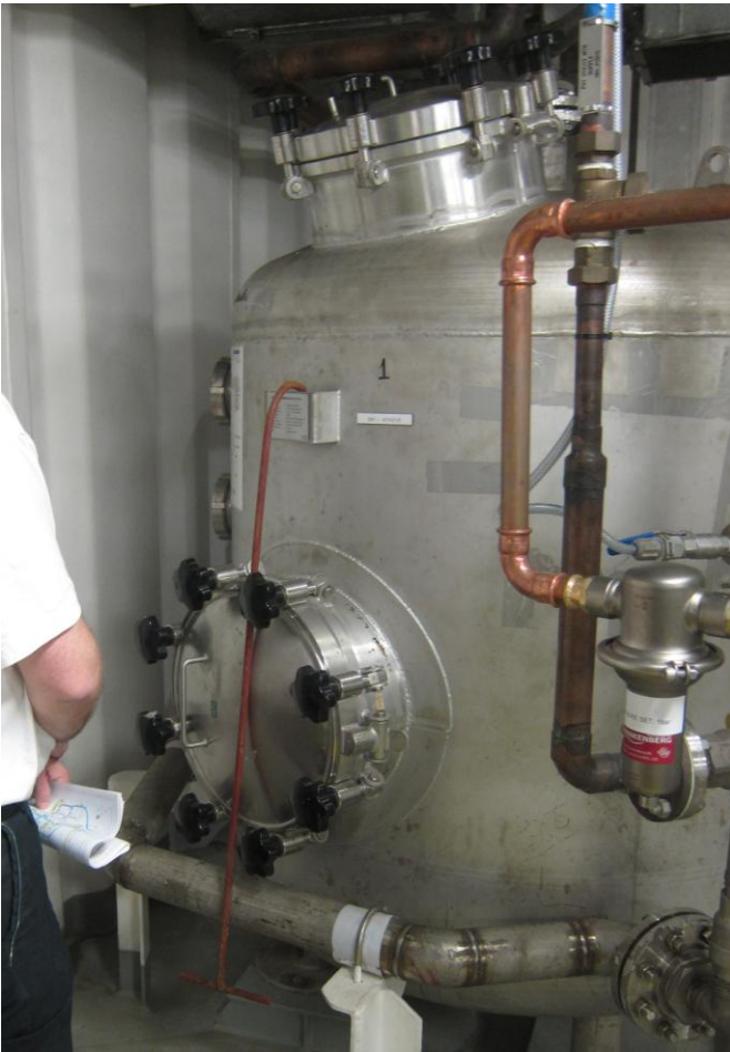
Figure 9.5: Also smaller tanks in the potable water system, like hydrophore tanks, calorifiers and alkalisng filters must have sufficient access for inside maintenance. The pictured tank is made of stainless steel and has sufficient manholes (Photo: Eyvind Andersen)
