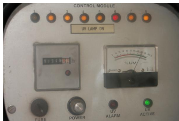
Figure 8.8: Control panel for UV-unit with eight UV-tubes. As both tube 6 and the signal lamp for tube 1 is defect, the UV-unit is not safe to use. The UV-intensity is still quite high. This may be due to clear water or long distance between UV-sensor and the defect UV-tube (Photo: Eyvind Andersen)
