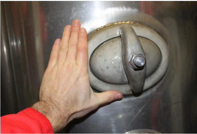
Figure 5.5: Alkalisating filters, hydrophore tanks and calorifiers are often supplied with access openings of such a small size that the tanks are impossible to clean (Photo: Eyvind Andersen)
