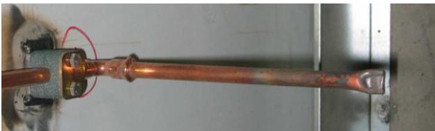
Figure 5.2: During the construction process it is important that pipe systems are not contaminated. The picture shows how pipe ends are secured by being compressed (Photo: Bjørn Løfsgaard)
