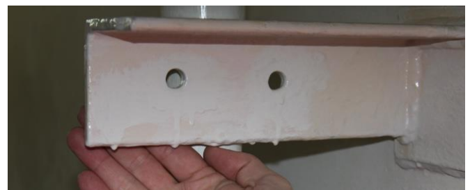
Figure 9.11: Picture from a tank where incorrect coating has resulted in corrosion and need for touch ups. Coating applied wrongly and too thick on cold steel increases the risk for microbial growth, and may cause unpleasant odour and taste from tank coating (Photo: Eyvind Andersen)
