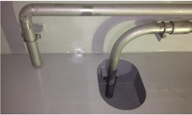
Figure 9.4: Tank suction (left) is elevated a few centimetres from the tank floor, whilst a drain suction pipe in the pump well in the middle makes it easy to empty the tank (Photo: Eyvind Andersen)
