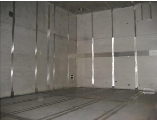
Figure 9.1: Approximately 4 metres high potable water tank in stainless steel with no obstructing internal structures. Such tanks are easy to clean, with no problems with applying and maintenance of coating (Photo: Bjørn Løfsgaard)
