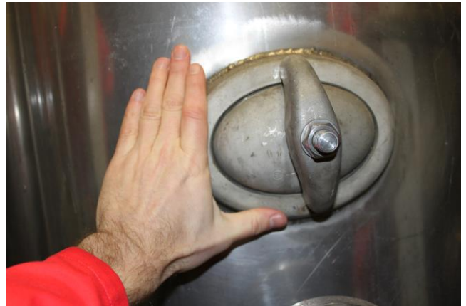
Figure 5.5: Alkalising filters, hydrophore tanks and calorifiers are often supplied with access openings of such a small size that the tanks are impossible to clean (Photo: Eyvind Andersen)
