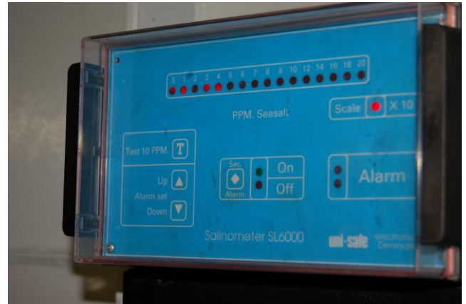
Figure 6.8: A conductivity meter automatically measures salt content in produced water and dumps it if the 6 mS/m limit is exceeded (Photo: Eyvind Andersen)
