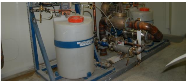
Figure 5.7: A marked and protected chlorine tank with easy access (Photo: Eyvind Andersen)
