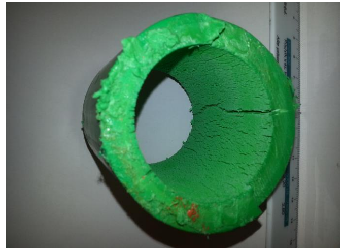
Figure 9.20: Hot water pipe damaged because of lacking expansion tank and too high pressure and temperature in the hot water system (Photo: Johan Ljungqvist)
