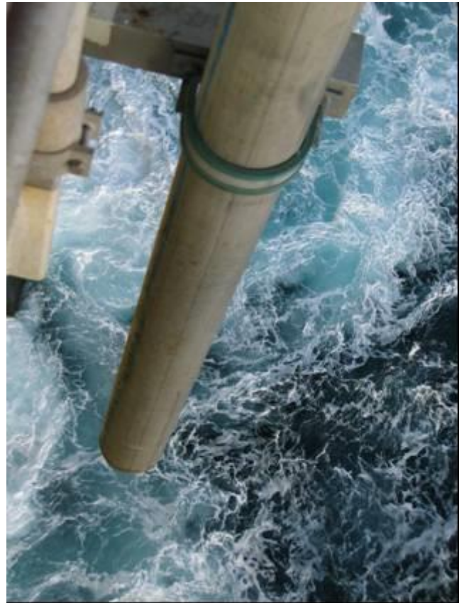
Figure 7.9: When flush valve and the bunkering hose have corresponding diameters the system can be flushed with maximum pressure. (Photo: Eyvind Andersen)
