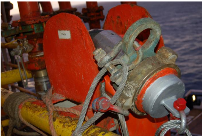
Figure 7.4 Bunkering hose with safely secured end-cap (Photo: Eyvind Andersen)
