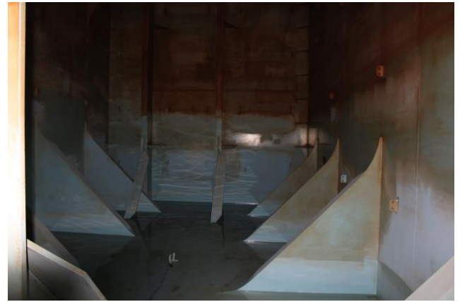
Figure 5.3: This potable water tank is high and lacks internal platforms for easy cleaning. This has resulted in insufficient cleaning. The walls are clean up to 2 metres and very dirty above 4 metres (Photo: Eyvind Andersen)
