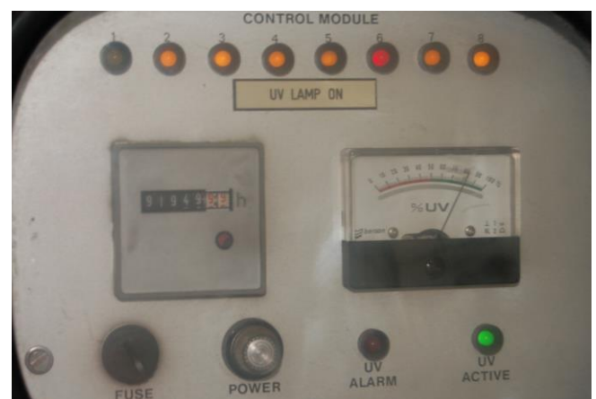
Figure 8.9: Control panel for UV unit with eight UV lamps. As both tube 6 and the signal lamp for tube 1 is defect, the UV unit is unsafe. The UV intensity is still quite high. This may be due to clear water or long distance between UV sensor and the defect UV lamp (Photo: Eyvind Andersen)
