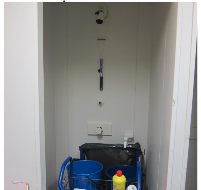
Figure 9.13: This shower is not in use, and is used for storage. Water in such pipes will be at room temperature, and there is a growth potential for Legionella and other microbes. This water may then contaminate the rest of the piping. Piping that is not in use should be eliminated, alternatively flushed weekly (Photo: Eyvind Andersen)
