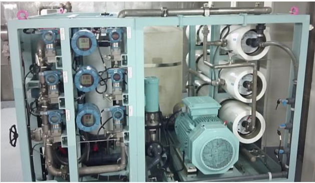
Figure 6.7: Reverse osmosis unit. The membranes lay coiled within the white tubes on the right (Photo: Eyvind Andersen)
