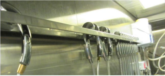
Figure 9.23: Shower hoses and heads are problem spots for Legionella growth due to low temperatures after mixers combined with stagnant water when not in use. Here growth is prevented through drying of the equipment (Photo: Arild Tolo)
