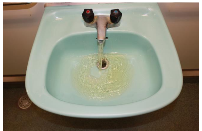
Figure 4.3: Discoloured water due to corrosion (Photo: Eyvind Andersen)
