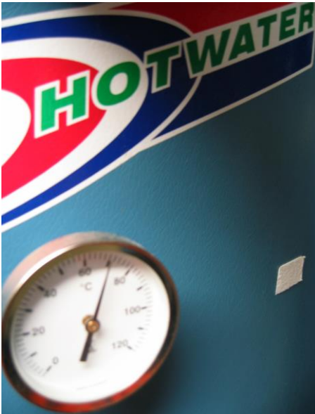
Figure 9.21: Legionella can be prevented by keeping the cold water cold and the hot water hot (Photo: Eyvind Andersen)
