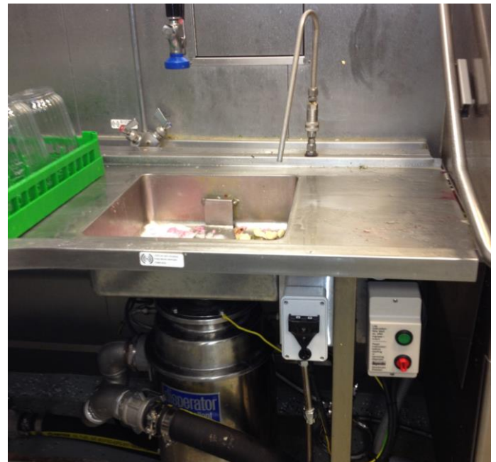
Figure 9.16: Full air gap of type «AA» is the best way of eliminating contamination from other systems supplied with potable water. Here water is supplied to a food grinder via pipe above the sink to the right (Photo: Eyvind Andersen)
