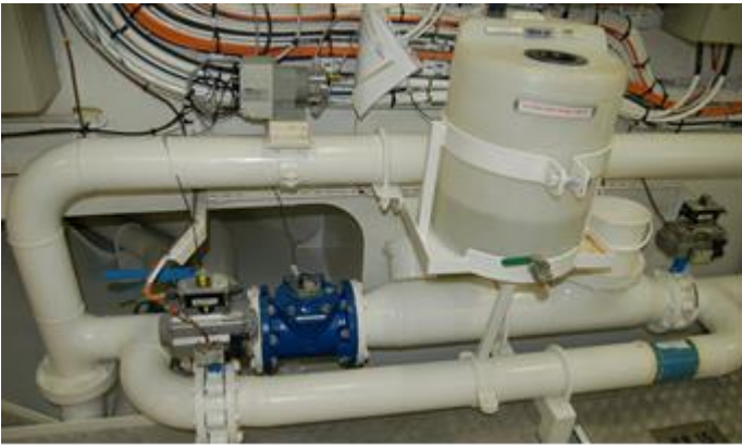
Figure 8.3: Flow meter-controlled chlorination unit (Photo: Eyvind Andersen)
