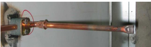
Figure 5.2: During the construction process it is important that pipe systems are not contaminated. The picture shows how pipe ends are secured by compression (Photo: Bjørn Løfsgaard)
