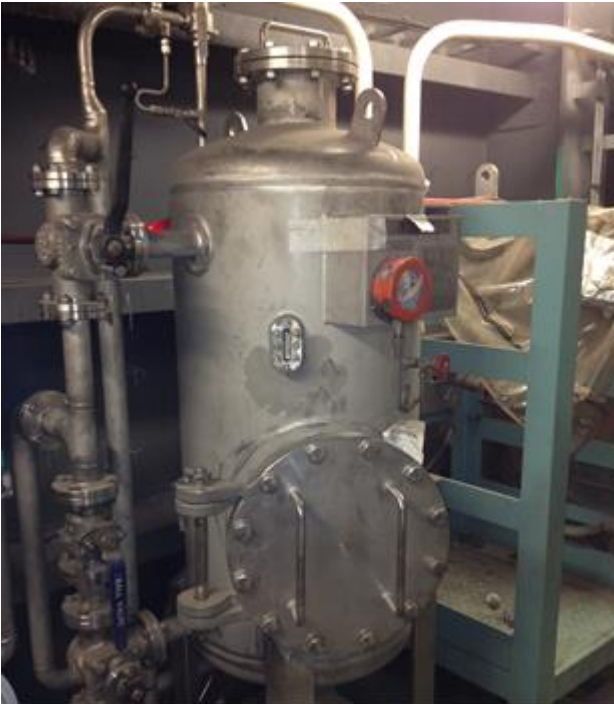
Figure 9.6: Also smaller tanks in the potable water system, like hydrophore tanks, calorifiers and alkalisng filters must have sufficient access for inside maintenance. The pictured tank is made of stainless steel and has sufficient manholes (Photo: Eyvind Andersen)
