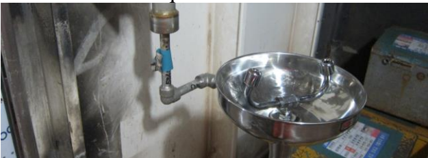
Figure 9.15: Due to slower (and laminar) flow in the large pipe than in the small pipe supplying an eye-wash station, biofilm will grow more easily in the bigger pipe (Photo: Eyvind Andersen)
