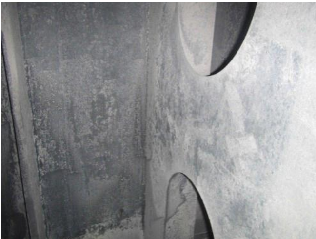
Figure 9.7: «White rust» in a potable water tank, is deposits of zinc carbonate. The tank is coated with a product that contains zinc, and that can be used in the pH interval 5.5 to 10. At higher pH, problems with deposits and high zinc levels in the water can occur. In this case poor pH management is the source of the problems, as the measured pH around 11 was far beyond the max limit of 9.5 in the potable water regulations. (Photo: Tjarda den Dunnen)
