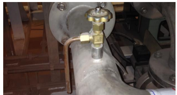
Figure 5.8: Short and self-draining test tap with sufficiently small pipe diameter. The short distance from main pipe to valve eliminates stagnant water. By placing the outtake on the upper half of the pipe, trapping of particles is avoided. A shorter sample point end would have eased sample point disinfection (Photo: Eyvind Andersen)
