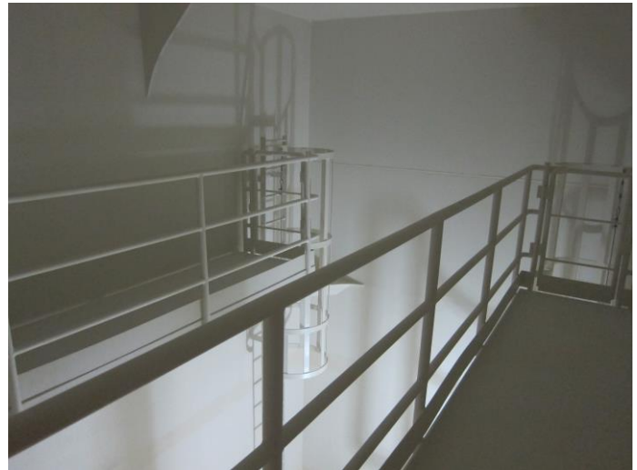
Figure 9.2: Access platforms aid maintenance in tanks over 4 metres high. Internal structures in tanks should be minimised to enhance circulation and minimise maintenance. Circulation is achieved by placing the inlet in one upper corner of the tank, whilst the outlet is placed in the opposite lower corner (Photo: Eyvind Andersen).
