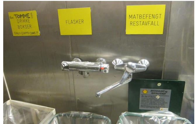
Figure 9.22: A sink has been removed whilst pipes and fittings remain, leaving dead ends where Legionella may have good growing conditions and later infect the rest of the potable water system (Photo: Eyvind Andersen)
