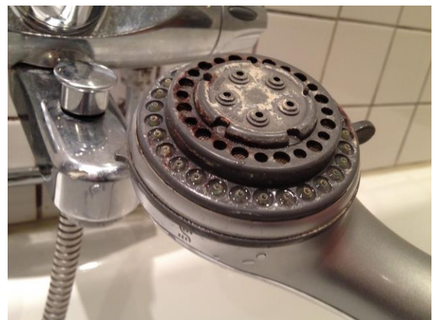
Figure 9.24: Such biofilm is a consequence of insufficient cleaning. Microbes have ample possibility for growth (Photo: Eyvind Andersen)
