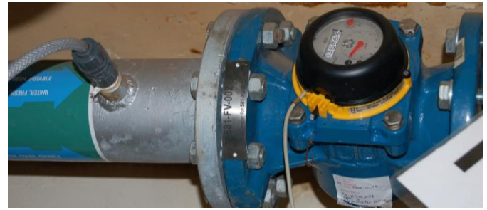
Figure 7.7: The flow meter display is visible to the right, and the chlorine hose and dosing point to the left (Photo: Eyvind Andersen)
