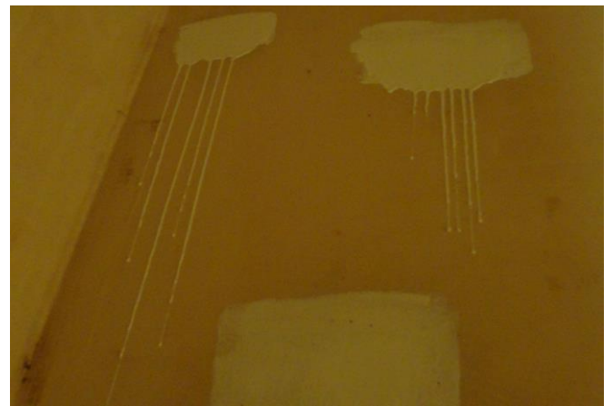
Figure 9.10: Incorrect coating. A roller has been used instead of a round brush, and the coating has been used on too large areas and in a far too thick layer (Photo: Bjørn Løfsgaard)
