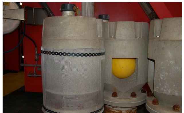
Figure 9.3: Protect air vents for potable water tanks. The picture shows vents safeguarded with floating ball and fine mesh corrosion material. The picture is taken on a newbuild prior to marking (Photo: Eyvind Andersen)
