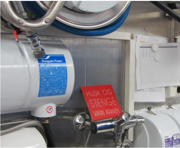
Figure 9.19: A hose station where water is leaking between the hot and the cold water when the mixer is left in open position and the hose is not in use. A sign to close the mixer is not a barrier against such leaks (Photo: Eyvind Andersen)
