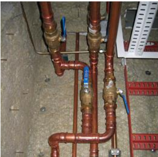
Figure 4.7: Corrosive water in copper pipes can result in excessive copper content in the potable water (Photo: Bjørn Løfsgaard)
