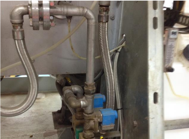
Figure 6.9: Evaporator with two independently controlled (blue colour) dumping valves (Photo: Eyvind Andersen)
