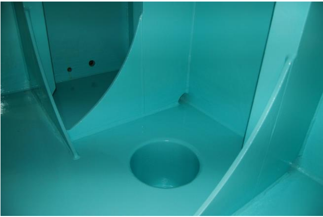
Figure 5.4: This tank has a drain well, and the stiffeners are placed vertically, with drain cavities against the tank floor. Consequently the tank is easy to drain (Photo: Eyvind Andersen)
