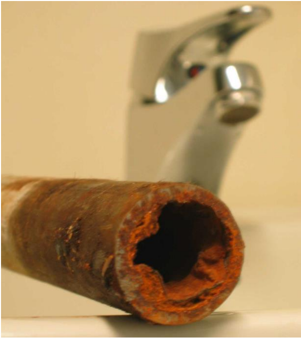
Figure 4.3: Corrosion clusters can result in poor water quality and clogging of pipes (Photo: Eyvind Andersen)
