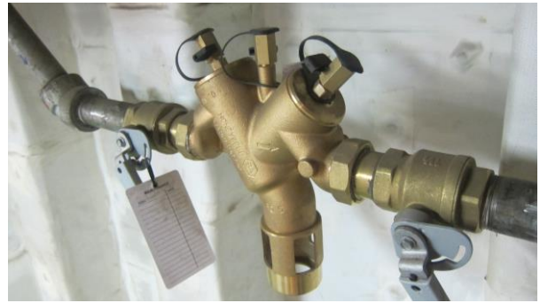
Figure 9.17: If other liquid carrying systems must be supplied with pressurised potable water, a BA type backflow prevention device gives the best level of protection. Note the 3 test points on top of valve. This valve needs to be fitted with a strainer and stop valves before and after for testing, and location over a drain is recommended, as it may open automatically (Photo: Eyvind Andersen)
