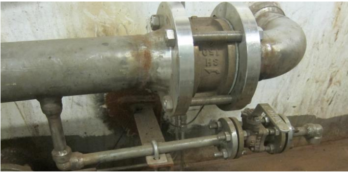
Figure 9.14: This test tap is not designed correctly, as it is too long and too big. In addition the outtake below the main pipe will increase the risk of biofilm formation, as dirt and particles will settle in the test pipe, and the water tests may not be representative (Photo: Eyvind Andersen)
