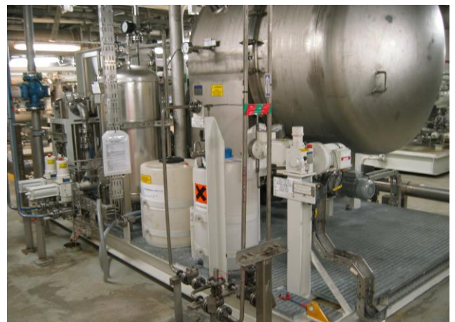
Figure 1.1: Potable water system with evaporator, scale inhibitor tank, chlorine tank, alkalising filter and UV units (Photo: Eyvind Andersen)
