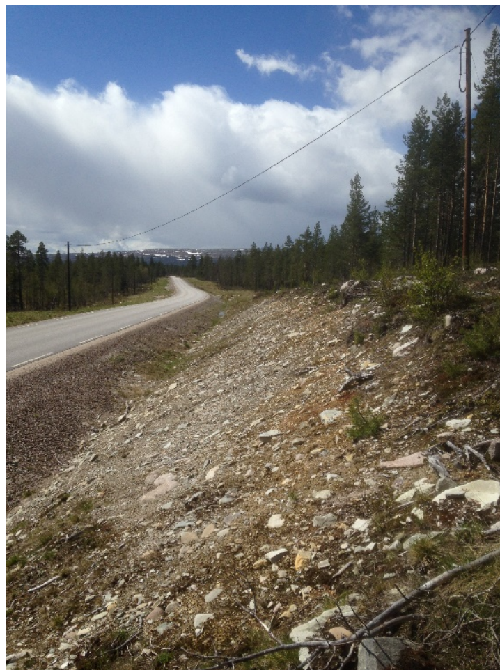
Figure 2.1.3-1: Re-use of topsoil to restore road verges after road rehabilitation approx. 600 m.a.s.l., Fylkesveg 2208 Engerdal municipality, Innlandet county. Photo: Line Rosef
